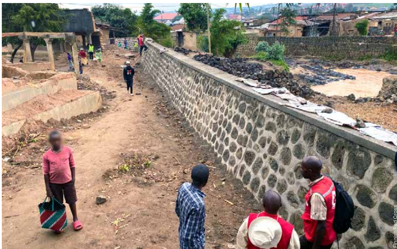
Flood retention wall was rebuilt after May 2023 floods in Mahoko cell, Kanama sector, Rwanda.
